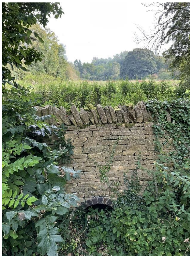
Photograph 4 - Partially collapsed culvert under the track, with upstream meadow in the background
