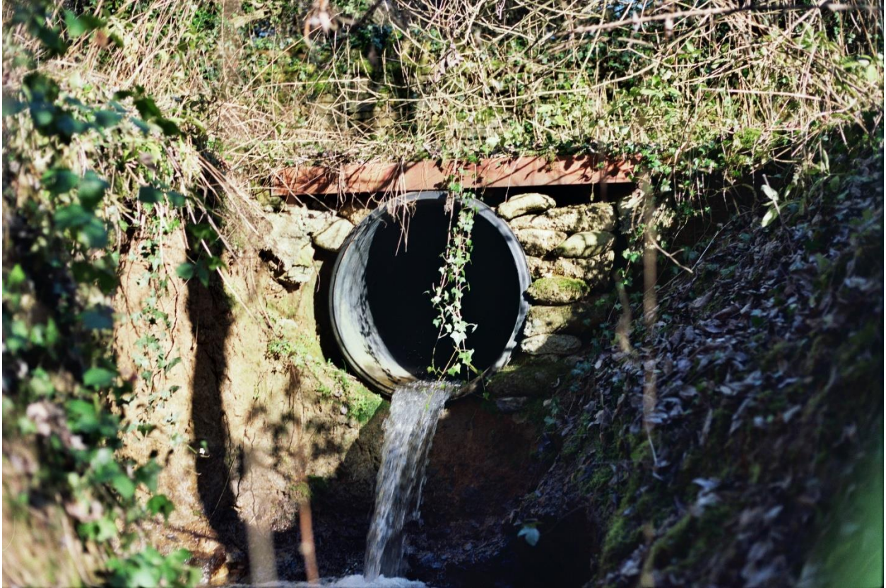
Photograph 2 - Pipe at the upstream end of the meadow (beneath the track from Church Lane)
